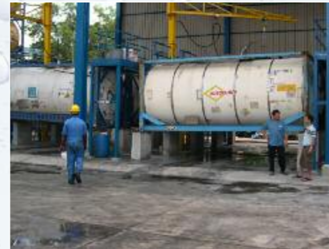
Tank cleaning station for interior cleaning of tank containers.
