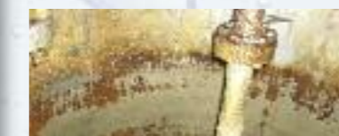
Dirty tanks with hardened products before cleaning.
