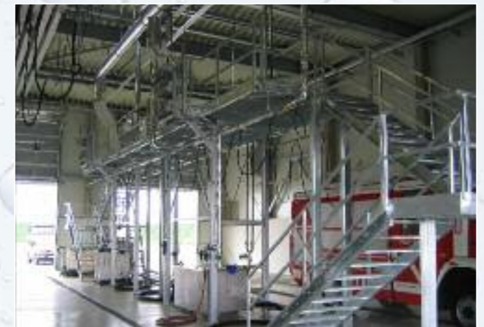
Tank cleaning station for interior cleaning in a cargo center.
