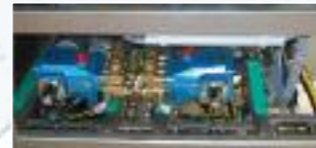
Multiple pump equipment.
